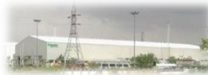
MV Transformer Vadodara (TBI)
